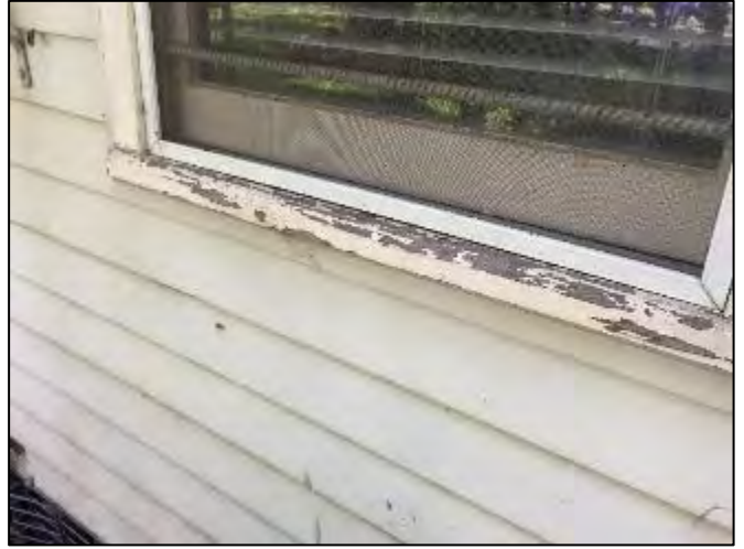
Plate 38 – Peeling paint around window frames at 60 Edmondson Avenue.
