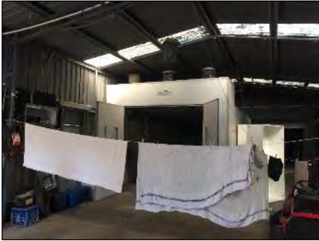
Plate 25 – Internal view of the large shed showing mobile spray booth.
